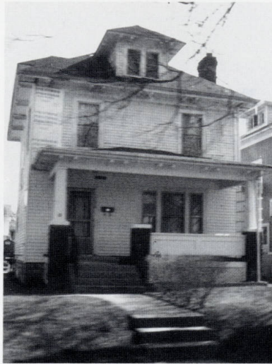
An older house in need of repair in Hilltop.
