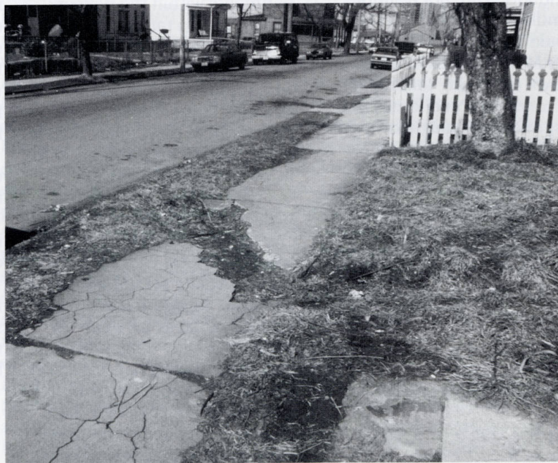
Poor maintenance of infrastructure poses a safety hazard and contributes to an atmosphere of decline.
