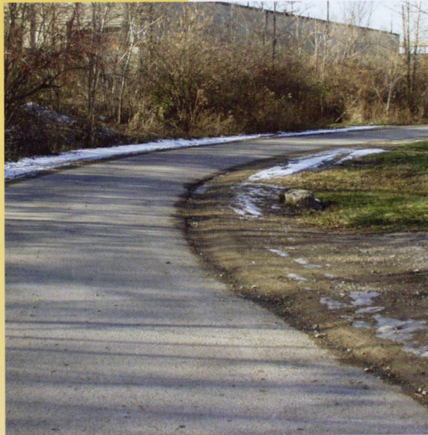
Wager Street: Insufficient roadway swales.
