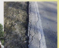
Roadway lanes lack shoulders
