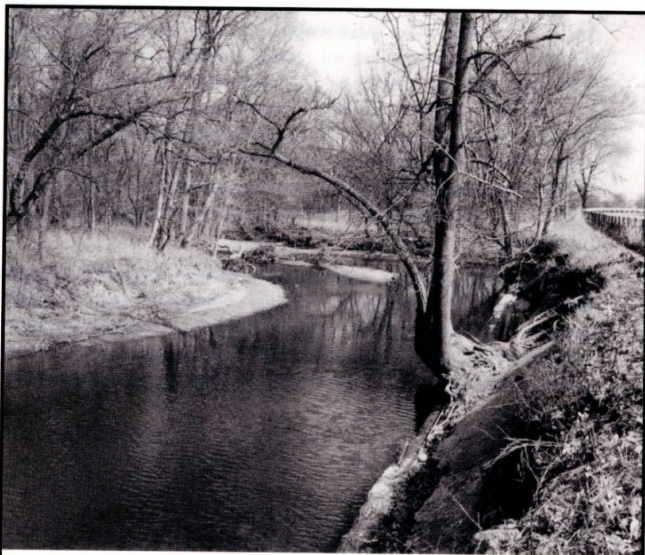
Stream bank erosion of Blacklick Creek along Shannon Road is a good reminder of the importance of preserving adequate watercourse open space buffers.
