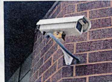
Facility Security Camera
